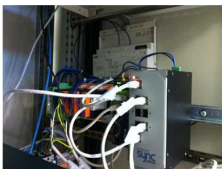
Figure 4 – Equipment installed for the demonstration project
